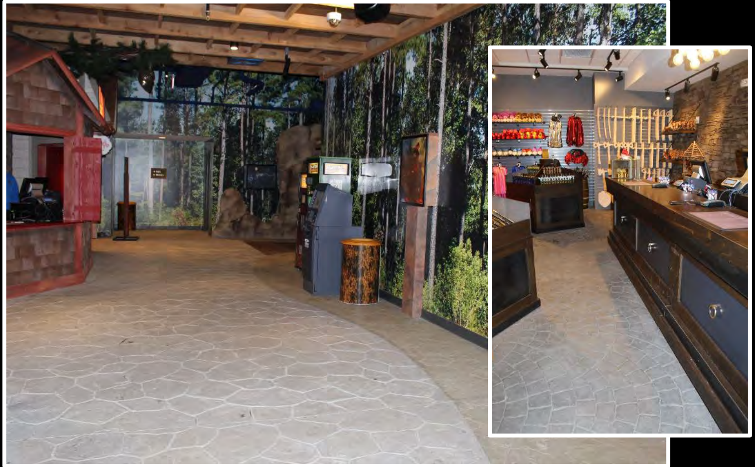
Project Location – Minnesota; Bomanite Toppings System – Bomanite Thin-Set Patterns Bomacron Small Sandstone, Bomacron Fishscale Belgian Block, Erosion Series Dried Earth Texture
